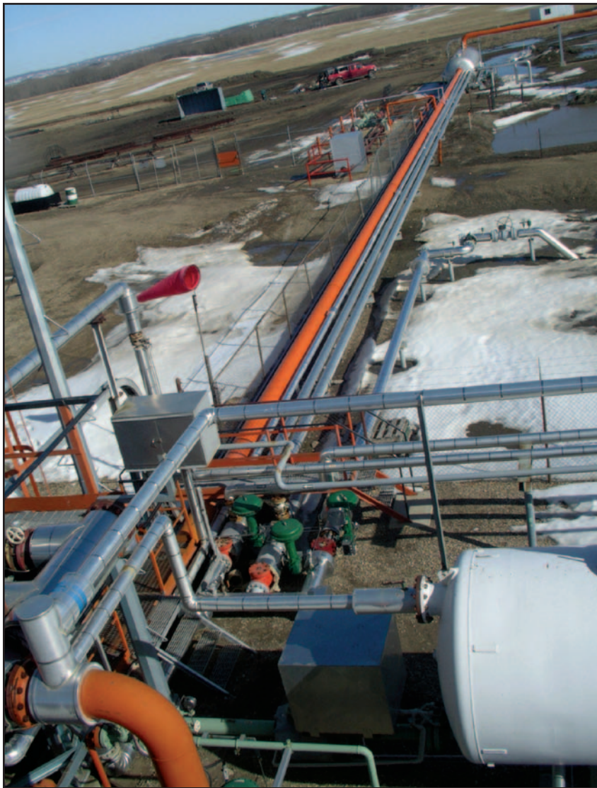
■ The gas compression facilities were constructed using the California model of the '40s, '50s and '60s. One feature of that design is the location of the auxiliary equipment, such as the coolers, filters, scrubbers and dehydrators, which are far away from the compressors.
