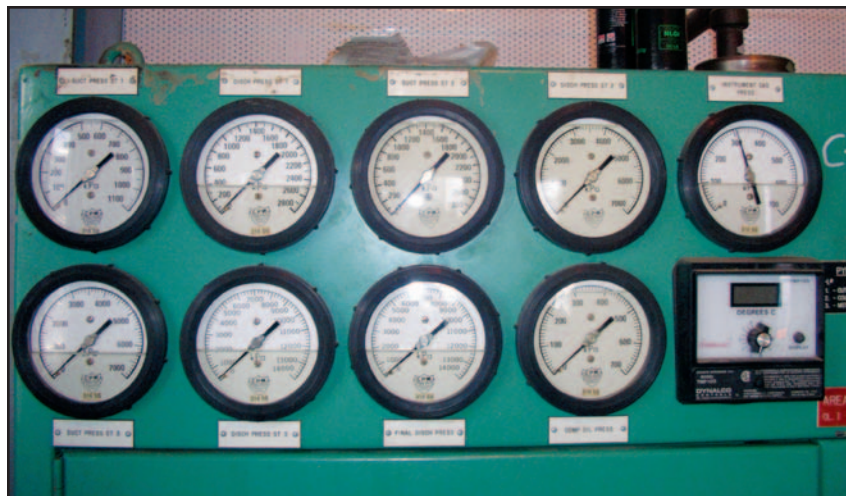
■ This compressor plant is operated manually. Each compressor has its own control system to monitor its operation, including speed control and safety shutdown. The control systems are independent and mainly pneumatic.
